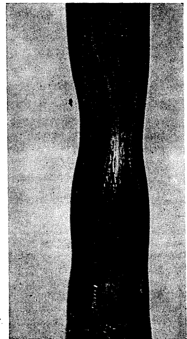
Figure 2. Typical example of tube from reboiler that had been crushed by explosion.
